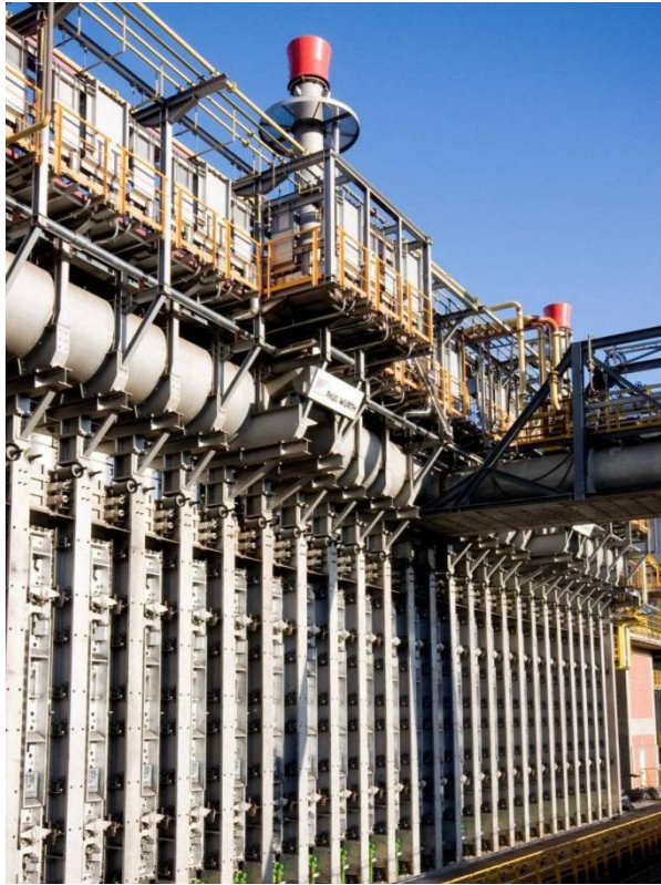
New coke oven batteries B3 and B1, Zentralkokerei Saar, Germany
