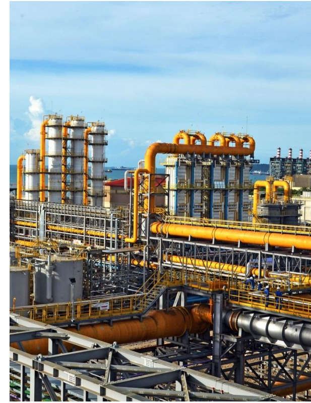
New coke oven batteries B1 and B2, including gas treatment plant, PT Posco Krakatau, Indonesia
