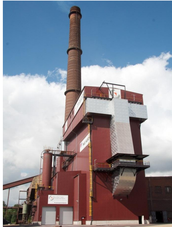
Sinterplant off-gas cleaning system, Salzgitter, Germany
